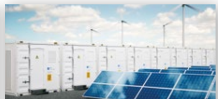
Battery energy storage systems (BESS)
